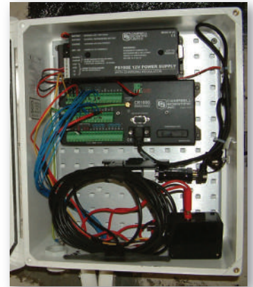
On-site Data-logging box
