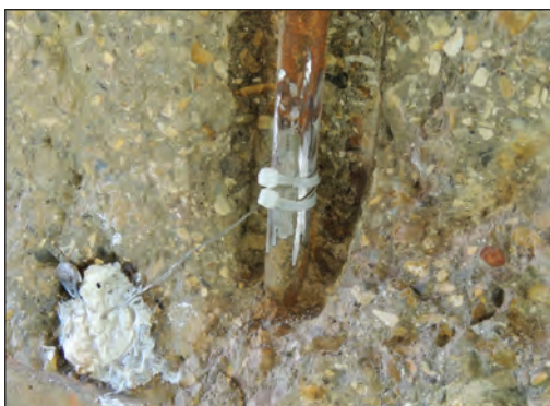
4. Connect the protruding titanium wire from the anode to the clean reinforcing steel rebar with a cable tie.
